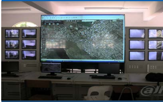
Mauritius Electricity Management Center
